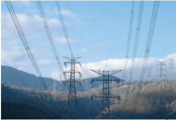
Overhead transmission line
